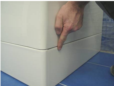
4. Offer panels to bath, and check height fitment and horizontal adjustment Ensure external panel radii are flush to edge of bath.
